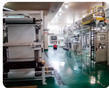
2011 Casting and coating lines installed.
